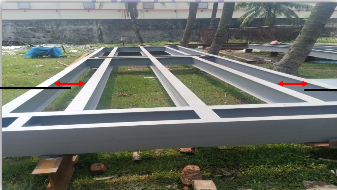
Picture: Mechanical Structure made by another company
